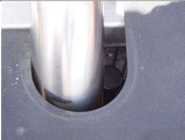
Photo 20-33: Pipe not centered
