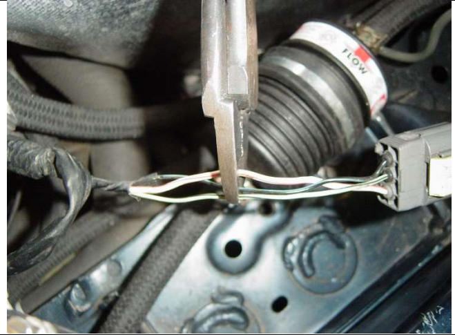
Photo 19-4: Wires cut about 2" from plug
