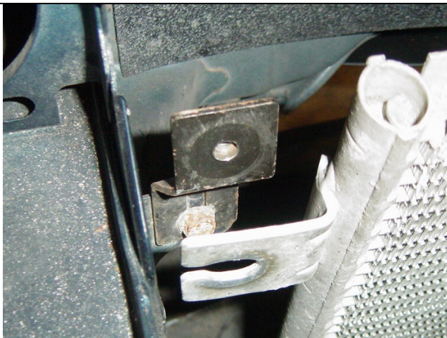
Photo 1-13: A/C condenser coil bracket one on each side
