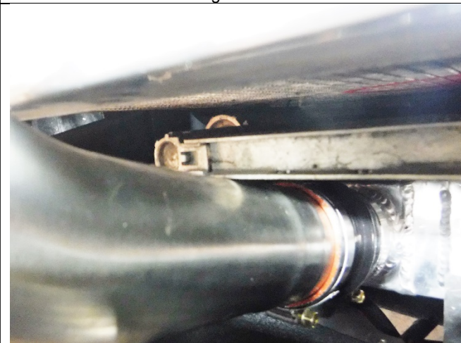
Photo 5-19: Top of condenser rub area at top
