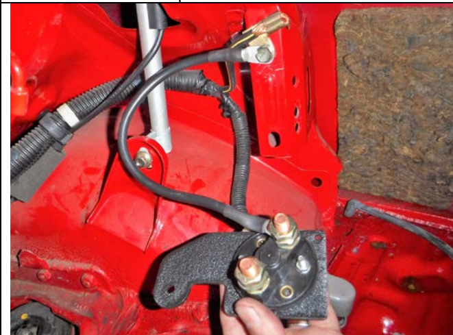
Photo 2-3: Ground strap attached to disconnect switch
