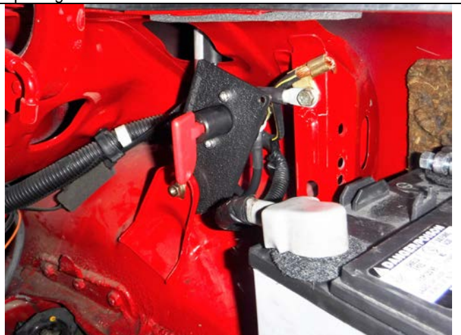
Photo 2-12: Disconnect key installed
