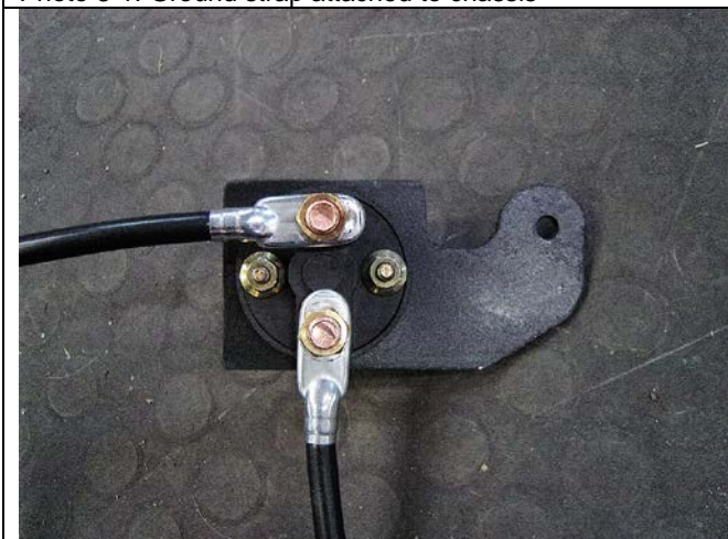
Photo 3-3: New ground strap attached to disconnect switch
