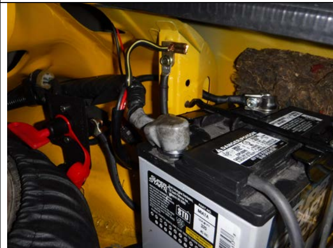
Photo 2-11: Battery connection complete
